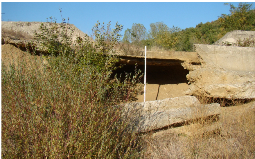
Figure 5 Apron undermining affecting 10% of the apron, having a depth of 3.0 m and an intensity rate of 0.3 of the structure 30B0.5 located on Bremenea Valley (the direct slopes of Danube)
