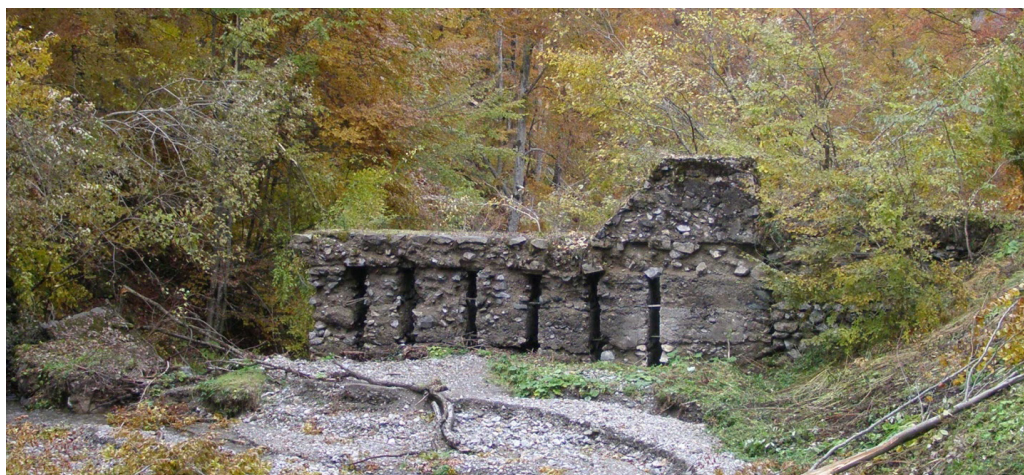
Figure 2 Multiple damages (wall wing and spilled area breaking, body abrasions, guarding wall breaking etc.) occurred during the exploitation of dam 90MF6.0 placed on the riverbed of Lungsor stream (Crişul Repede Watershed)
