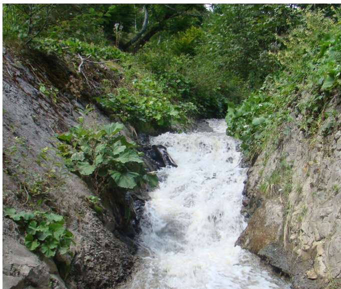
Figure 12 Drain channel 10KM137 on Plaic Stream (Tisa Watershed) built on 1965 and repaired on 2005
